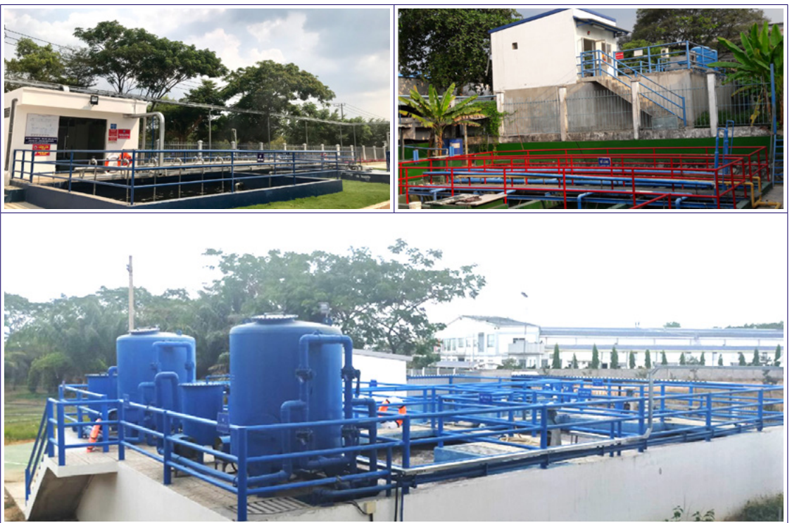
▲ Waste Water Treatment Plant (WWTP)
