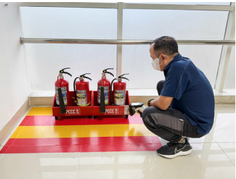
RFID-based fire equipment scanning system
